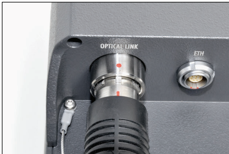
Figure 136: Correctly aligned fibre connectors
